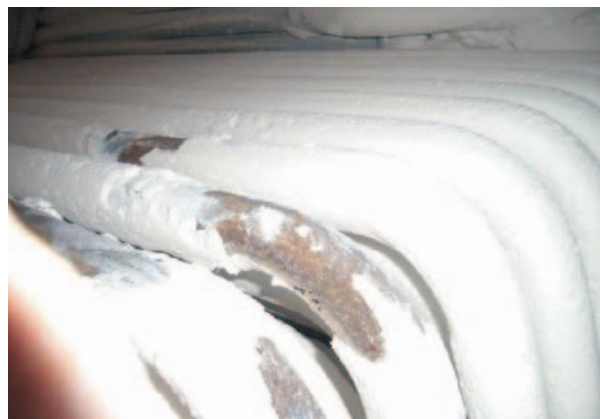
Figure 2: Boiler tubes coated with SiO 2 . Photo courtesy of Applied Filter Technology.
